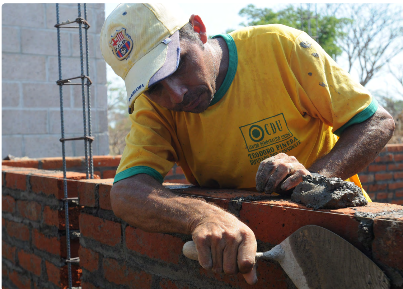
House reconstruction in El Salvador on a higher foundation to be resilient to floods
